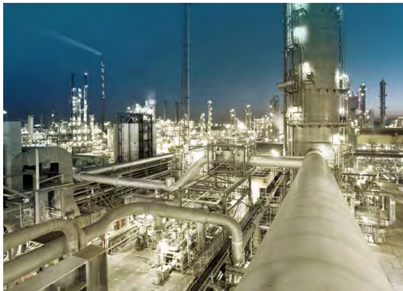
Power-teK loose wool Cryo LWC was used to insulate a new minus 160°C coldbox developed by BASF and Linde Engineering in Ludwigshafen, Germany
