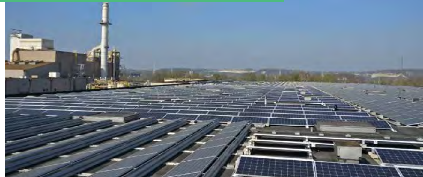
A total of 6,000 photovoltaic panels have been installed at our plant in Visé in Belgium
